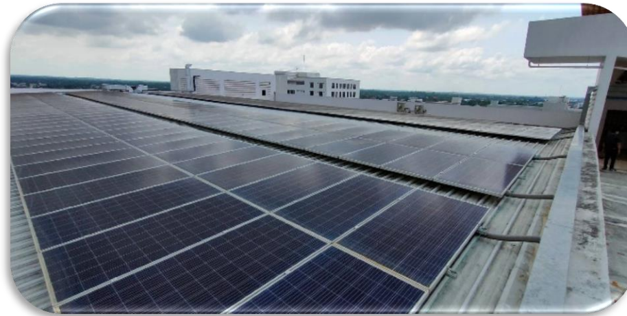
Solar Roof 304 KW
